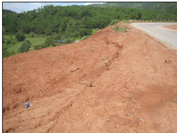
Figure (5) Slump in residual soil at the western part of Wetphyuye
