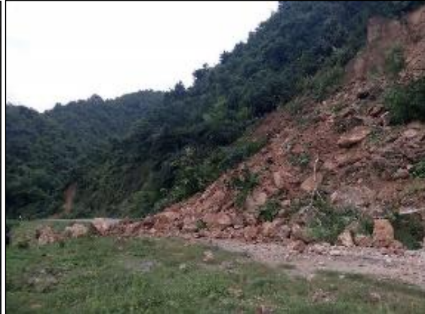
Figure (3) Debris flow at the eastern part of Yebokson
