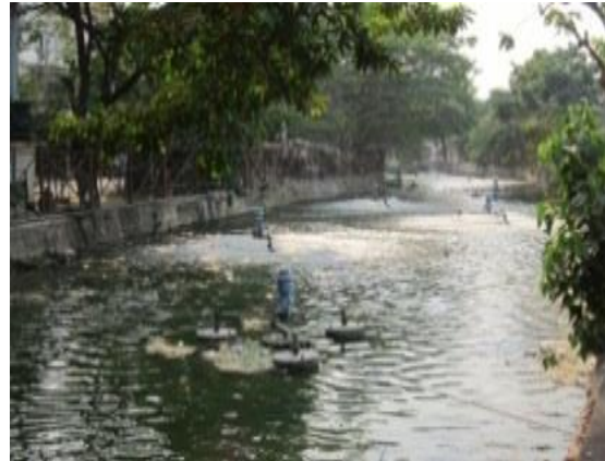
Figure 7. Surface Aerator on the water canal
