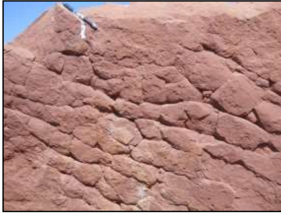
Fig. (3) Dessication cracks on thin-to medium-bedded red sandstone of Kalaw Formation south of Yegauk village ( 20^{\circ} 7' 4.99'' N 96^{\circ} 44' 38.33'' E)
