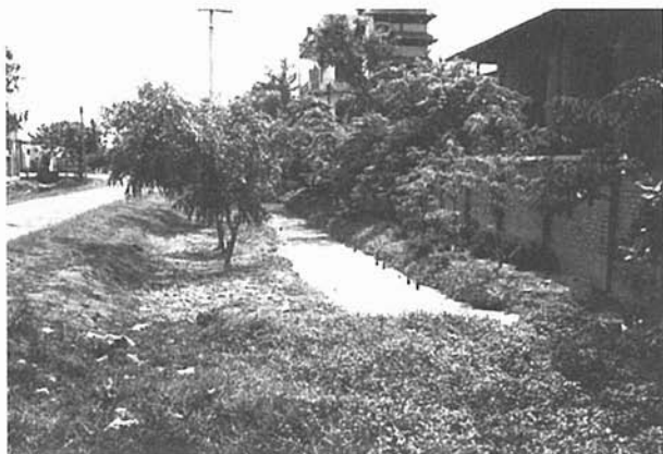
Fig. 8: A part of a drain in Shwepyitha industrial zone, which is block with weed and waste into which the wastewater from adjacent liquor factory are directly disposed of without any treatment. (Photo: Zin Nwe Myint 2002)
