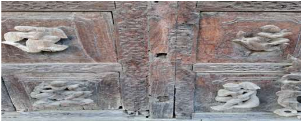
(Fig.3, damaged by Insect pests)
