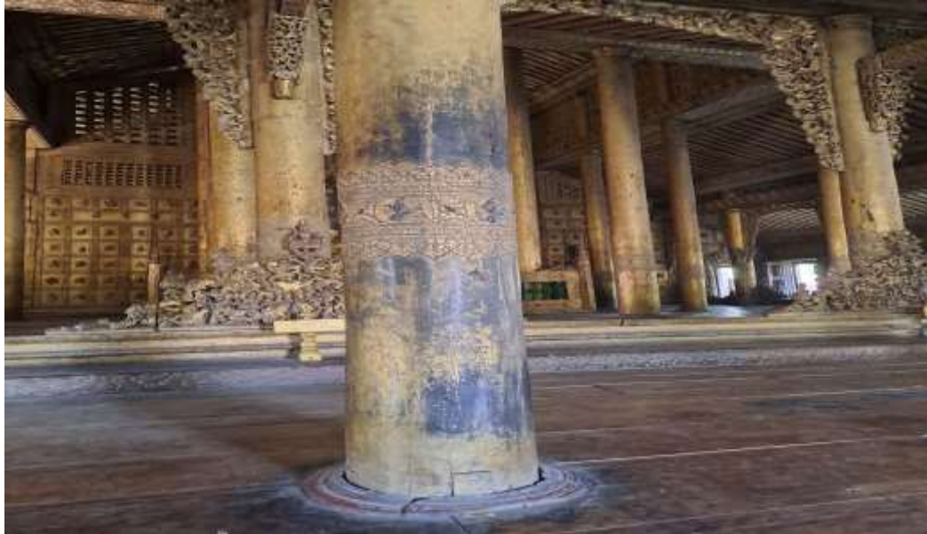
(Fig.1, damaged by man-made activities)
