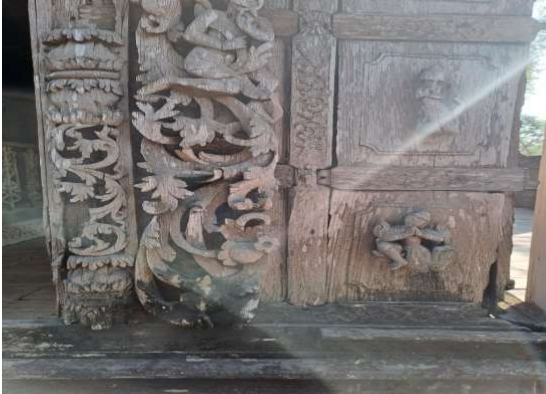
(Fig.2, damaged by weather)
