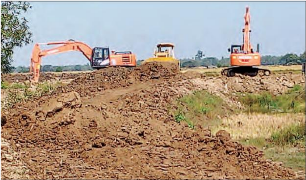
Dam construction in Laputtar Township, Ayeyarwaddy Division Photo- Kyemon (The Mirror Daily)
